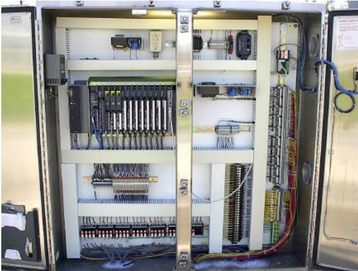
An example of PLC control panel
