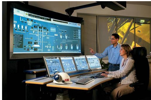
Central Control Room for all plants
